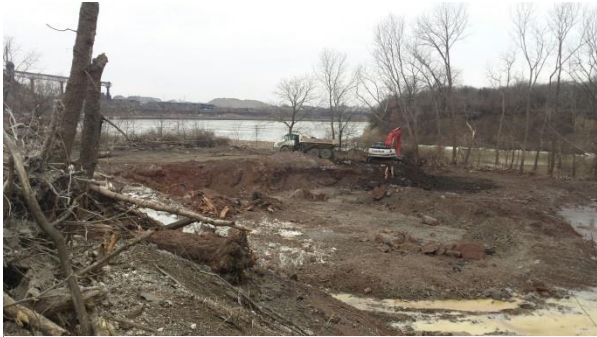
ODNR Rookery Restoration Project During Construction / Slag Excavation: Courtesy of City of Lorain
