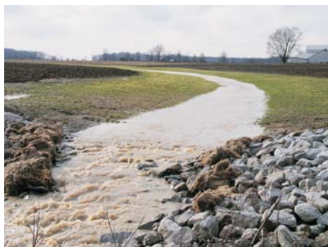
Completed grassed waterway project on private lands in Brighton Township. Agricultural producer constructed 3200 feet of waterway to control gully erosion as a result of concentrated storm water flow. Project funded through the USDA, Conservation Reserve Program. Rock rip-rap is installed at end of waterway to control subsidence where water enters main stream channel.
